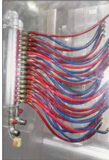
DME cooling manifold
